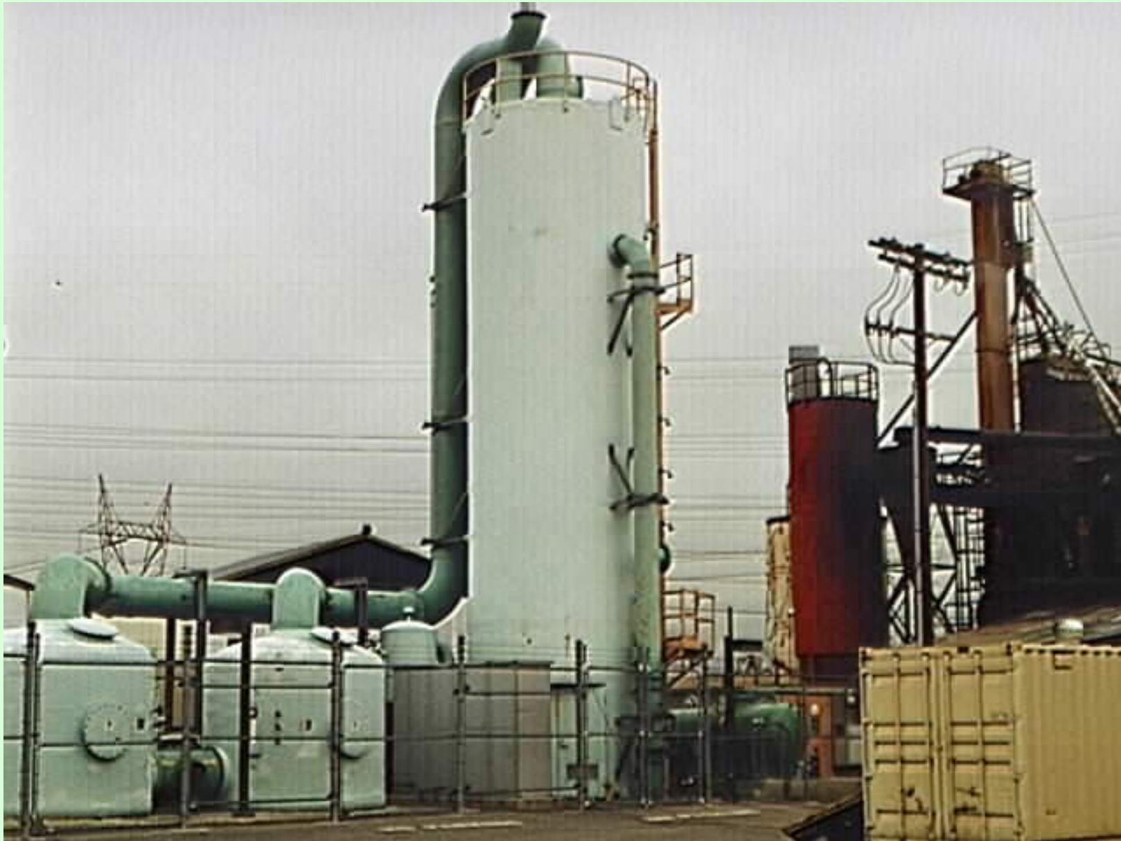
Source: Environmental Protection Agency, Region 9, San Fernando Valley, North Hollywood Treatment Plant, Air Stripping Tower, http://yosemite.epa.gov/r9/sfund/sphotos.nsf/0/7e416ed1a4259a7d88256612006c9b4c?OpenDocument/ . Accessed May 11, 2004.
